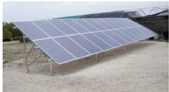
Figure 4. The photovoltaic array.
