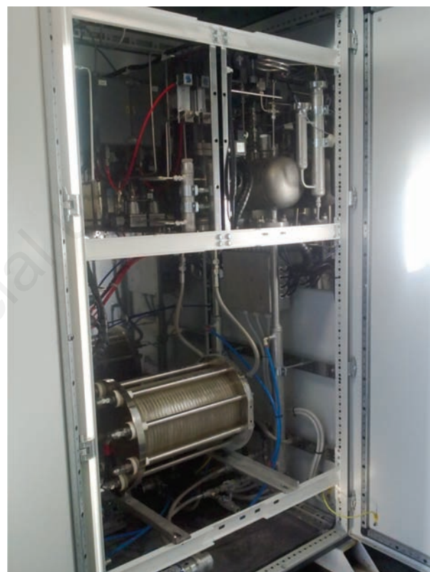
Figure 3. The electrolyser bank.
